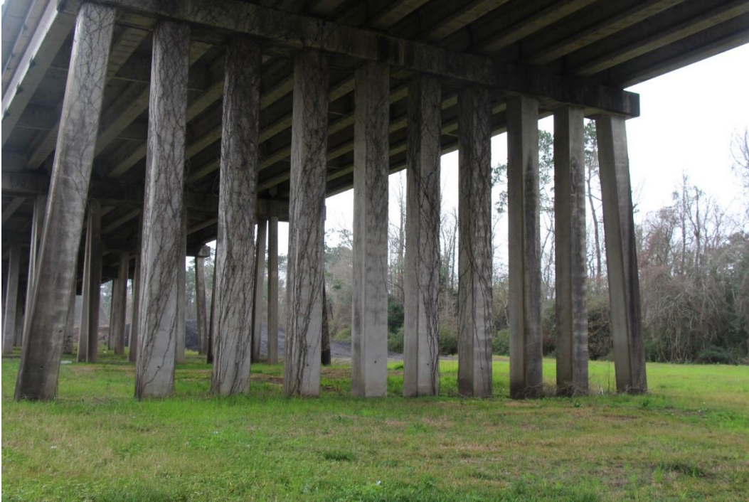
Condition Photo 9: Vines and vegetation growing on the concrete bent pile columns.
