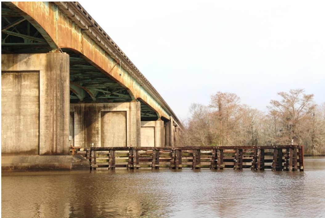
Condition Photo 18: East timber fender system.
