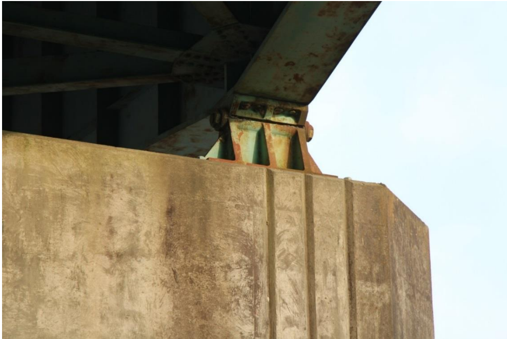
Condition Photo 15: Paint failure at the steel bearings of the main span, typical for all bearings.
