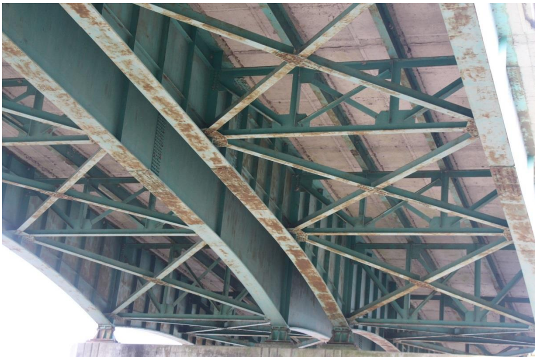
Condition Photo 12: Underside of main spans, steel plate girder paint failure.
