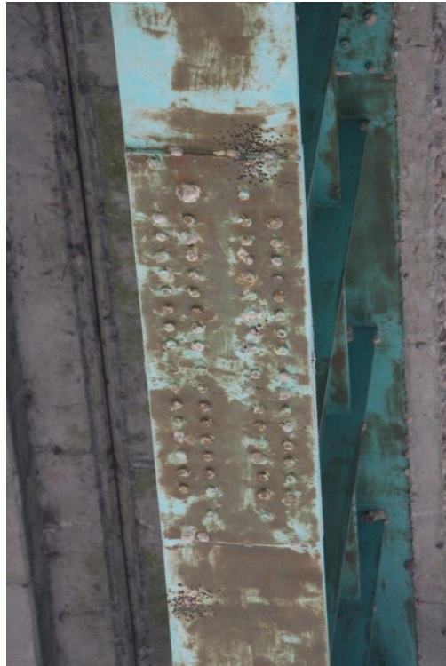
Condition Photo 13: Main span, steel plate girder field splice paint failure, typical at all splices.
