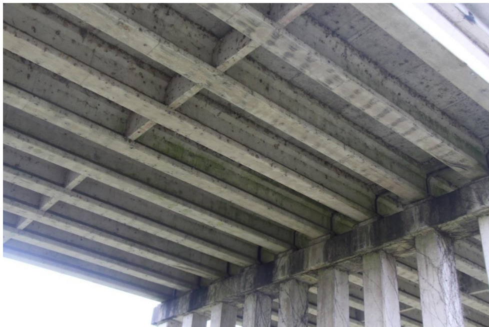
Condition Photo 6: Dirt dauber nests and efflorescence on the underside of the precast prestressed concrete beam approach spans.
