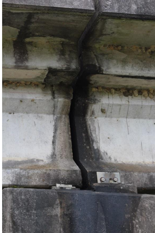
Condition Photo 5: Dirt dauber nests and water staining at the concrete approach bent caps.
