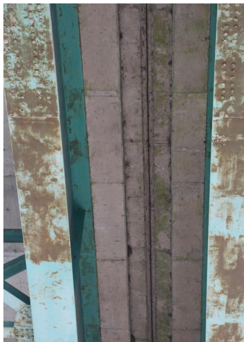
Condition Photo 14: Underside of joint between the northbound and southbound roadways exhibiting efflorescence and staining on the concrete deck underside.
