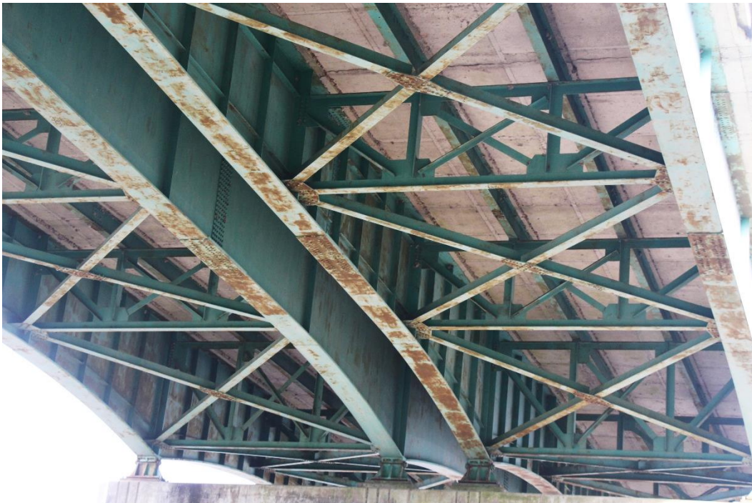
Character-defining Feature Photo 3: Design and construction of the steel plate girder and concrete girder superstructure. View of the underside of the steel plate girder main spans.
