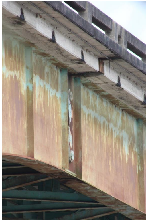
Condition Photo 11: Paint failure of the main span steel girder pin and hanger assembly, typical of all pin and hanger assemblies; also shows failure of paint system on steel girders.
