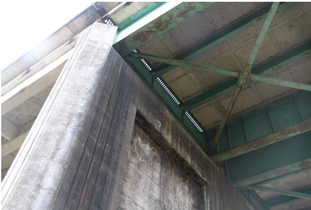
Condition Photo 16: Underside of finger-type expansion joint at the transition from the approach spans to the main span.
