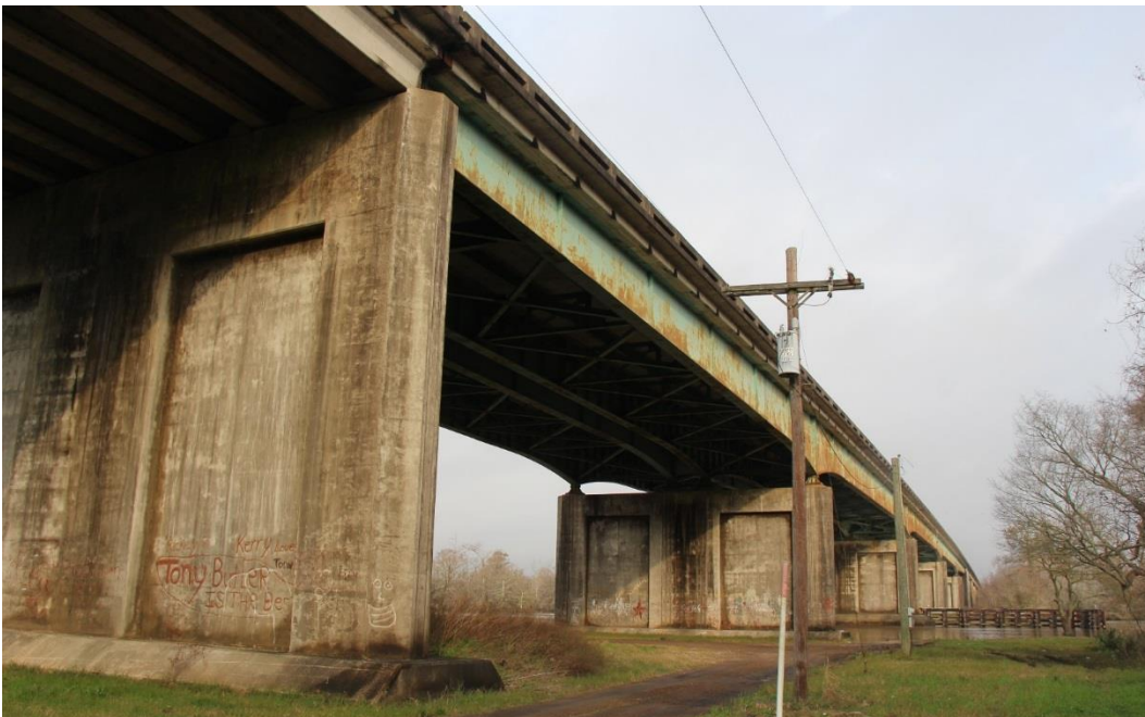
Condition Photo 10: Elevation view of the main span (five steel plate girder spans), showing piers 1 and 2, and showing failure of paint system in steel girder spans.
