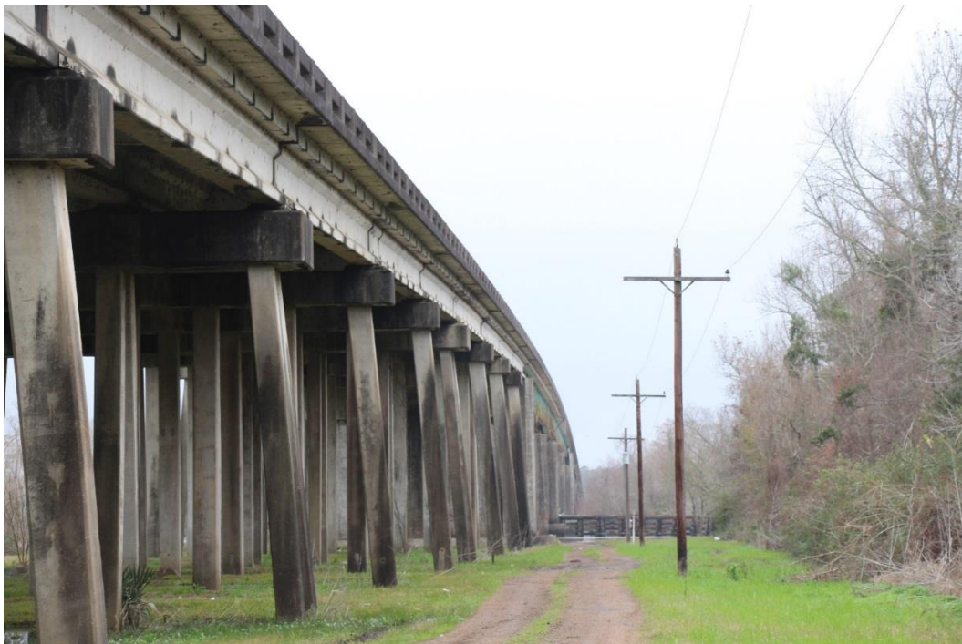
Condition Photo 8: Water staining on the approach span concrete pile bents.
