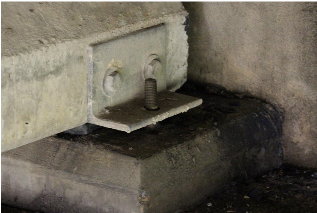
Condition Photo 4: Missing bolt at the concrete beam tie down at end bent 1, beam 7.
